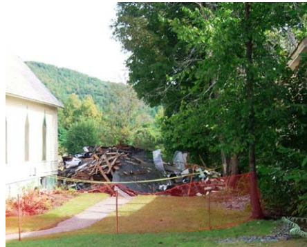
Gethsemane, Proctorsville parish hall destroyed. Photo by Thomas Ely
